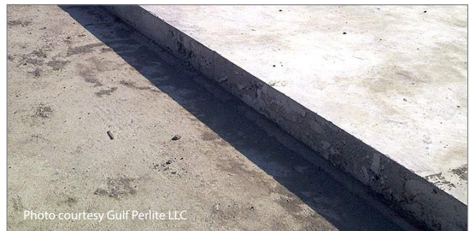
Top: Placing and screeding a perlite lightweight concrete roof deck. Above: Strong, smooth, monolithic surface of a perlite lightweight concrete roof deck installation.
