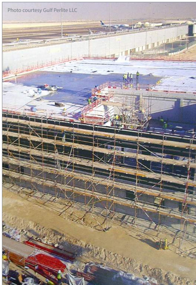
Figure 1 • Abu Dhabi Airport Terminal roofing with perlite lightweight insulating concrete stand-alone insulation.
